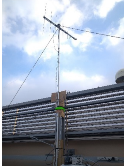
Figure 4c: Receiving-side equipment (Kyoto University Kizu Farm) Antenna
