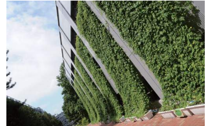
A “green wall,” which contributes to the reduction of building temperature and energy conservation
