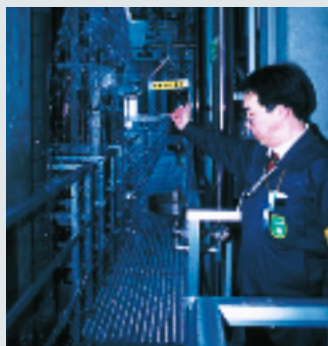
Inspection of emergency shower, a mandatory facility for each laboratory. It is located directly next to the emergency exit.
